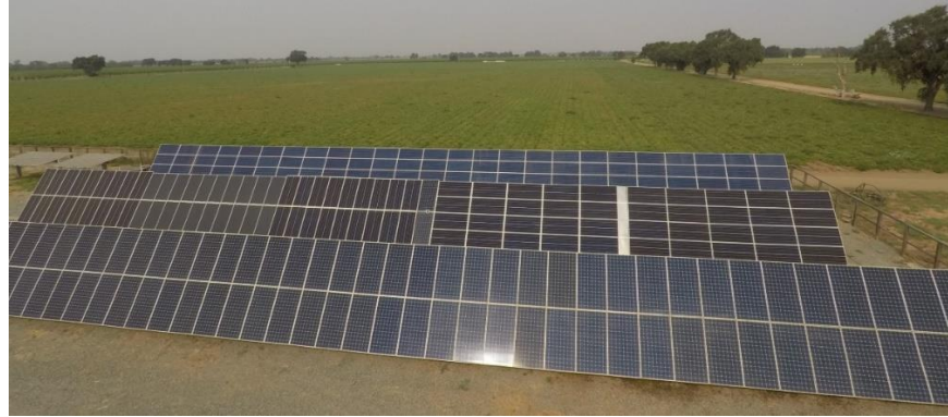
Figure 4.9. Single-axis tracking system installed at SunPower R&D Ranch in Davis, CA.
