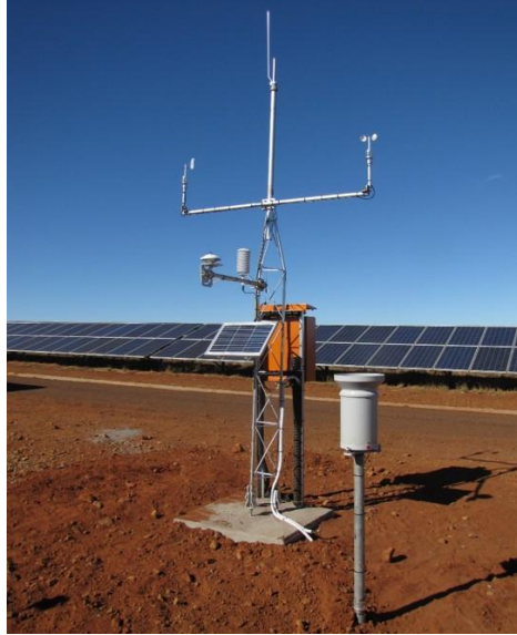
Figure 2.19. A SCADA weather station installed in Africa. (Figure from www. geosun.co.za )
